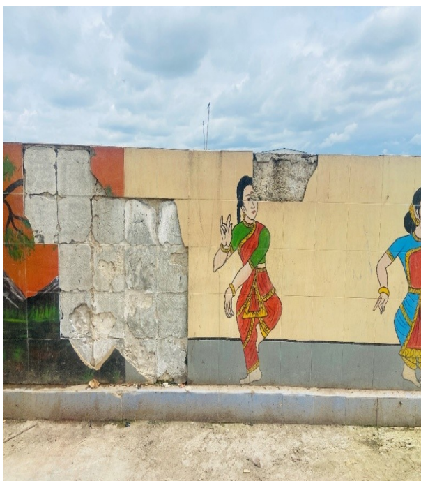
Issue of Wall Maintenance
